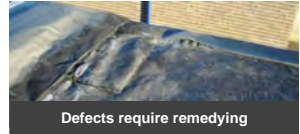
Defects require remedying
